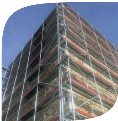
Radovi na Južnoj kuli / Reconstruction of the South Tower Izvor / Source: Arhiva JU PPM / Archive of PI NPM
